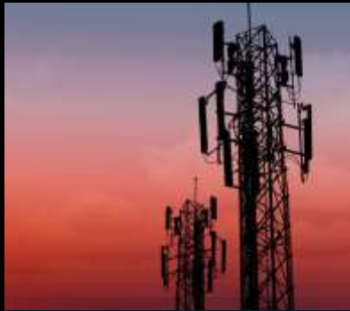
5G & Comms Infrastructure
